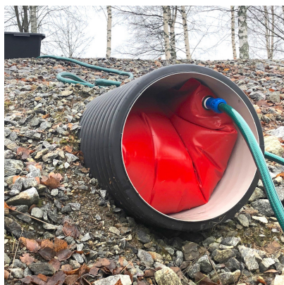
Road drums may need to be plugged
